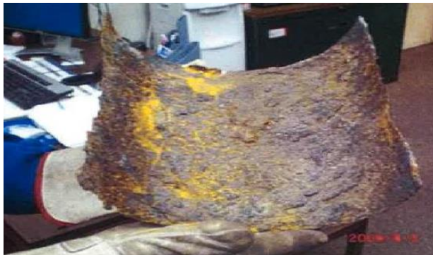
Welded Metallic Saddle Corrosion
