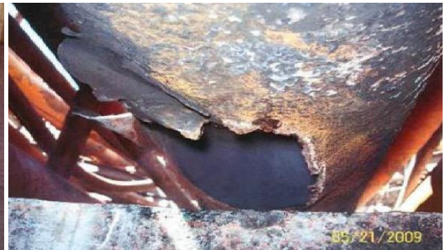
Welded Metallic Saddle Failure
