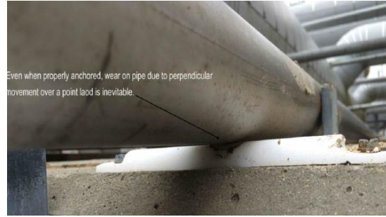
Plastic Rod Failure
